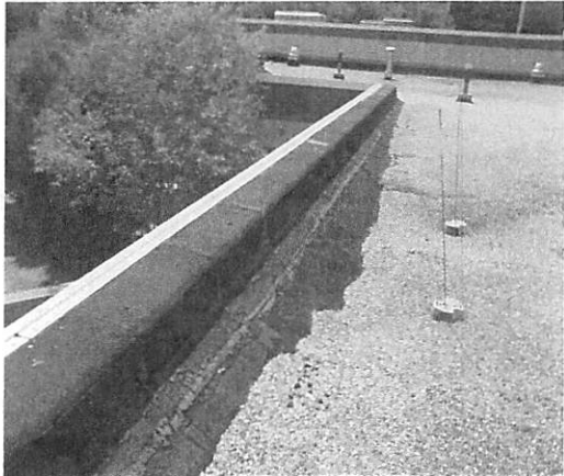
Photo #2: View of the uncoated wall flashings facing North on Section C
